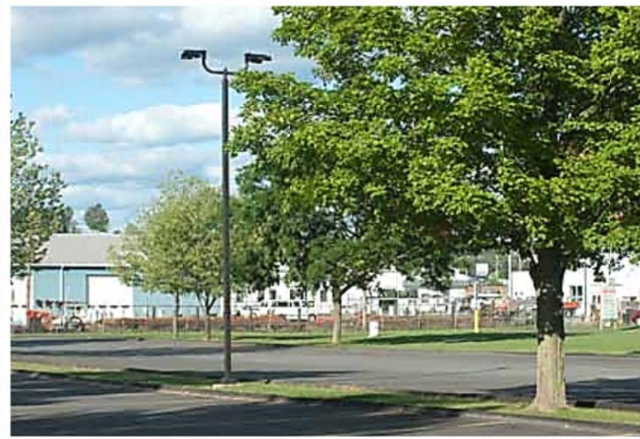
Two SL-90's on a pole.
